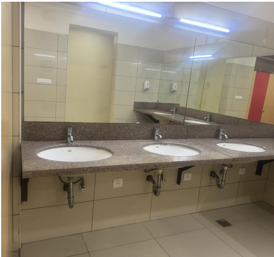
Picture2: Sensor based low faucets in MUJ washrooms
